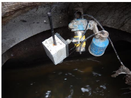
Level sensor with wireless transmission in a sewer (Photo: Frank Blumensaat, Eawag)
