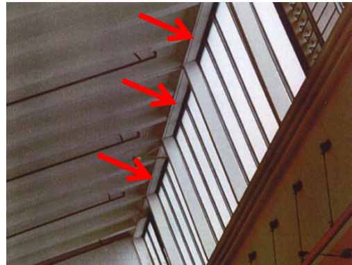
Figure 2: Detail of the inside of the building. The red arrows indicate the location of the steel plates. Photo was taken in the year 1992.
