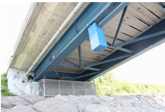
Figure 11: Underside of the bridge. The CFRP strips for the strengthening of the cross-direction are visible between the steel girders.
