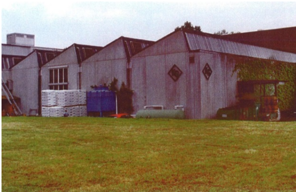
Figure 1: Industrial building in Kreuzlingen in Switzerland, which was strengthened in 1970 by means of steel plates.
