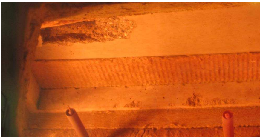
Figure 3. Second spall of specimen 1_Ref near southern support (after about 20 minutes in the fire).
